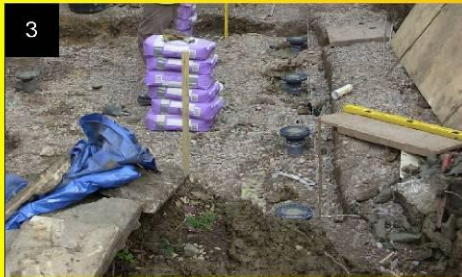
Levelling heads are fitted over the installed piles and the piles/heads infilled with a high strength grout.
