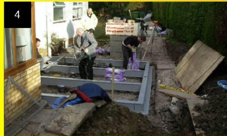
The Quickbase beam sections are then fitted together on top of the pile levelling heads. Reinforcement is added to the beams which are then infilled with a high strength grout.
