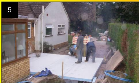
The final Quickbase site operation is to install the floor panels and trim to size.
