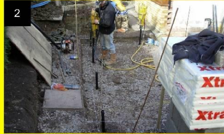
The piles for the extension had to be drive to a depth of 4.7m to protect against the influence of the adjacent trees. A total of 10 piles were installed.
