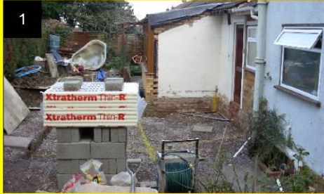
It was proposed to construction a kitchen extension on a Quickbase foundation for this property in Cheltenham. The photograph shows the site preparation following demolition of an existing structure.
