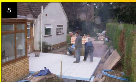
5 The final Quickbase site operation is to install the floor panels and trim to size.
