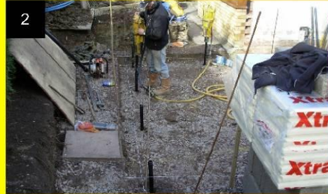
2 The piles for the extension had to be driven to a depth of 4.7m to protect against the influence of the adjacent trees. A total of 10 piles were installed.
