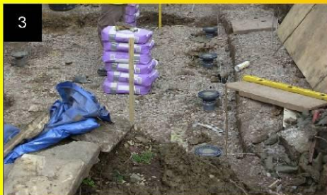
3 Levelling heads are fitted over the installed piles and the piles/heads infilled with a high strength grout.
