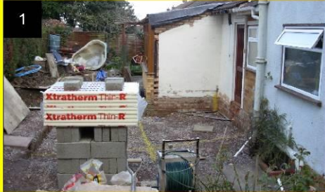
1 It was proposed to construct a kitchen extension on a Quickbase foundation for this property in Cheltenham. The photograph shows the site preparation following demolition of an existing structure.
