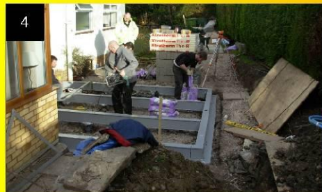
4 The Quickbase beam sections are then fitted together on top of the pile levelling heads. Reinforcement is added to the beams which are then infilled with a high strength grout.
