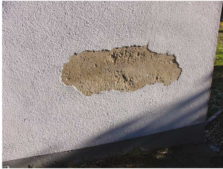
Figure 2: Adhesion of paint damaged by salts
