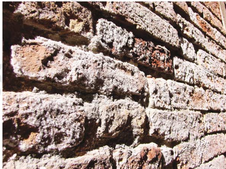
Figure 1: Salt-induced decay of brick masonry can be seen by the rounded corners. Salts have precipitated on the surface of the masonry as efflorescence
